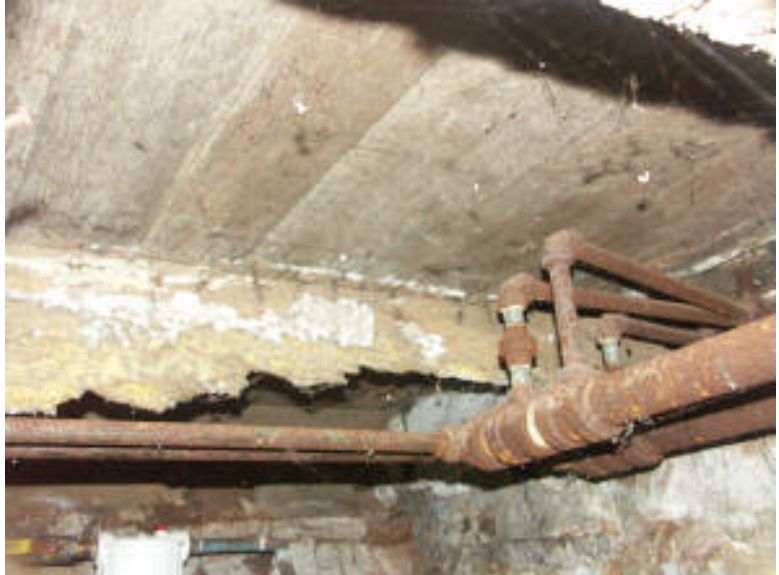
Photo 37. Damaged joist in center section, facing south.
