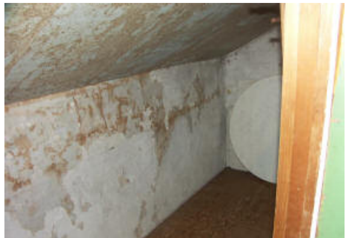
Photo 39. Dampness in attic of south section.
