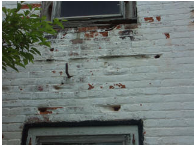
Photo 36. Deteriorating brick on south wall of main block.
