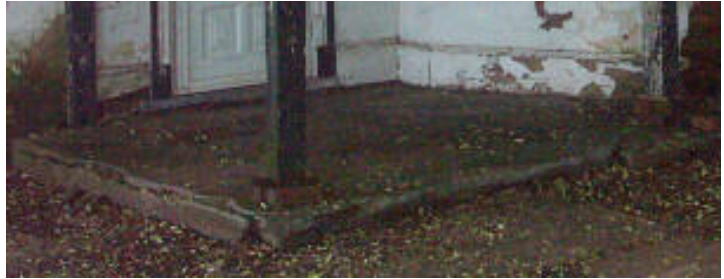
Photo 36a. View of the concrete pad on the porch, west elevation, showing deterioration.
