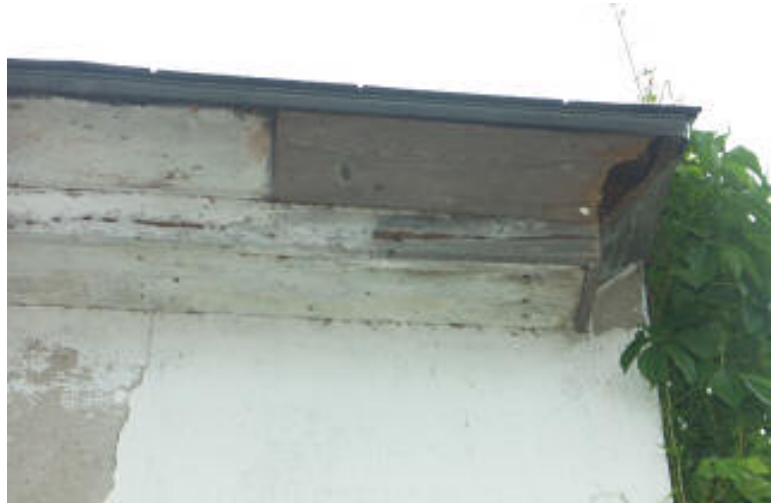
Photo 38. Damage to the cornice, south section.
