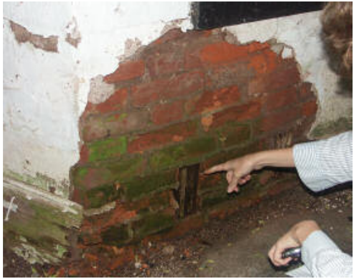
Photo 36b. Damage on the west elevation of bay window.
