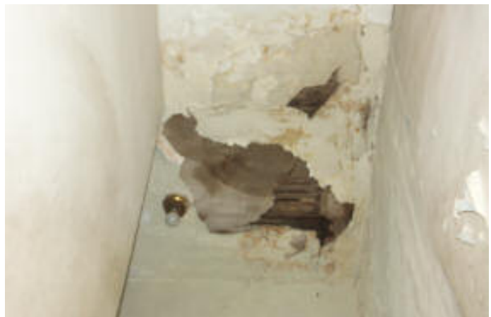
Photo 39a. Water damage in the hallway of the south section.
