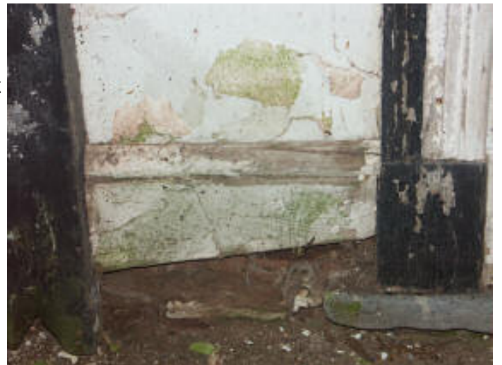
Photo 36c. Damaged baseboard molding on exterior wall, porch on west elevation.
