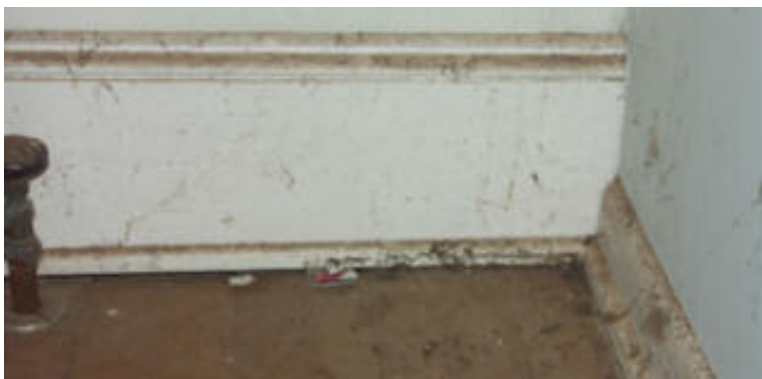
Molding 8. Junction of spiked baseboard molding and beveled molding, found on the second floor of the center section.
