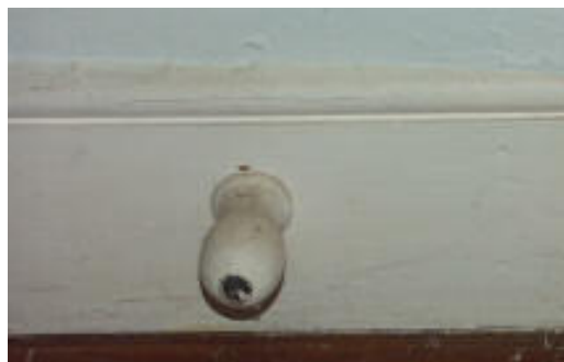
Molding 2. View of the earliest baseboard molding, found on the first floor of the center section.
