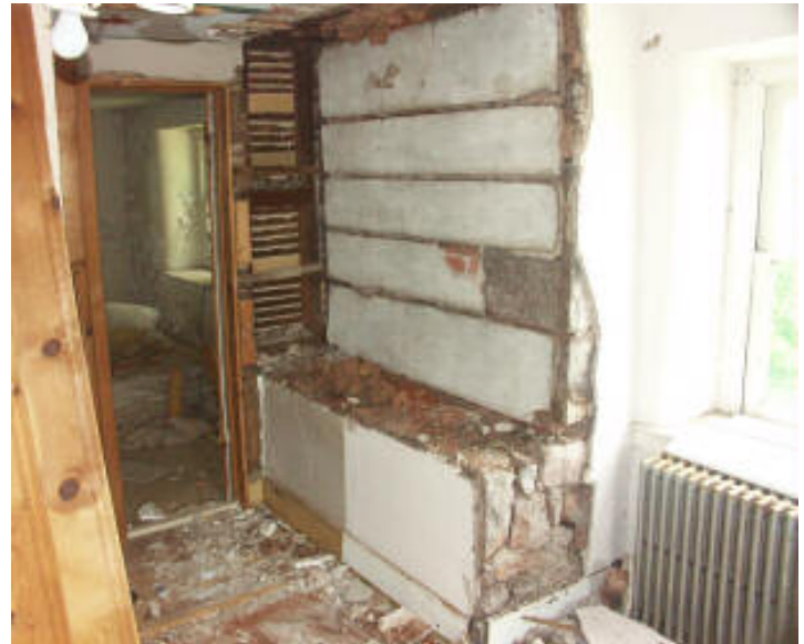
Photo 23. Remnants of chimney mass in Room N3.
