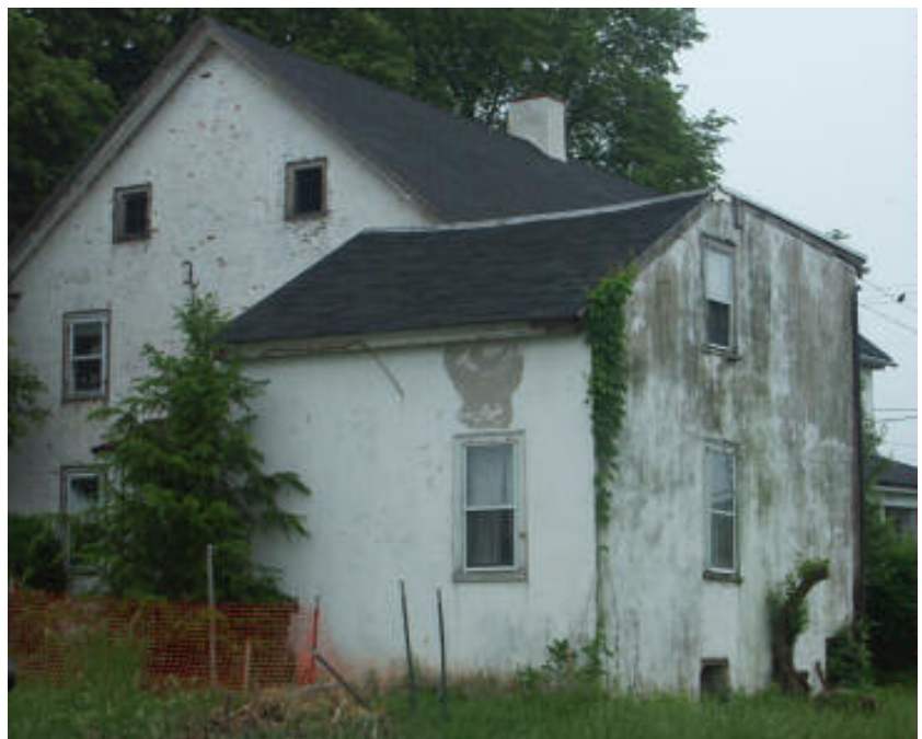
Photo 12. South section, facing northwest. The area under the flatter roof extent is the Connection.
