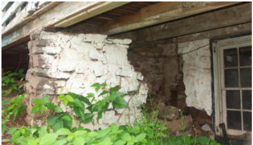
Photo 8. Stone wall supporting porch on east elevation; note structural failure.
