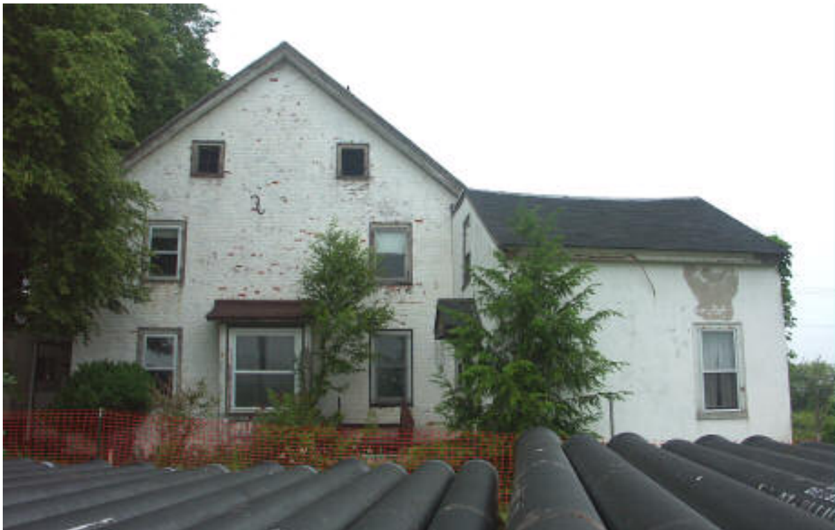
Photo 4a. South elevation of house, showing the main block (L) and the south section (R).
