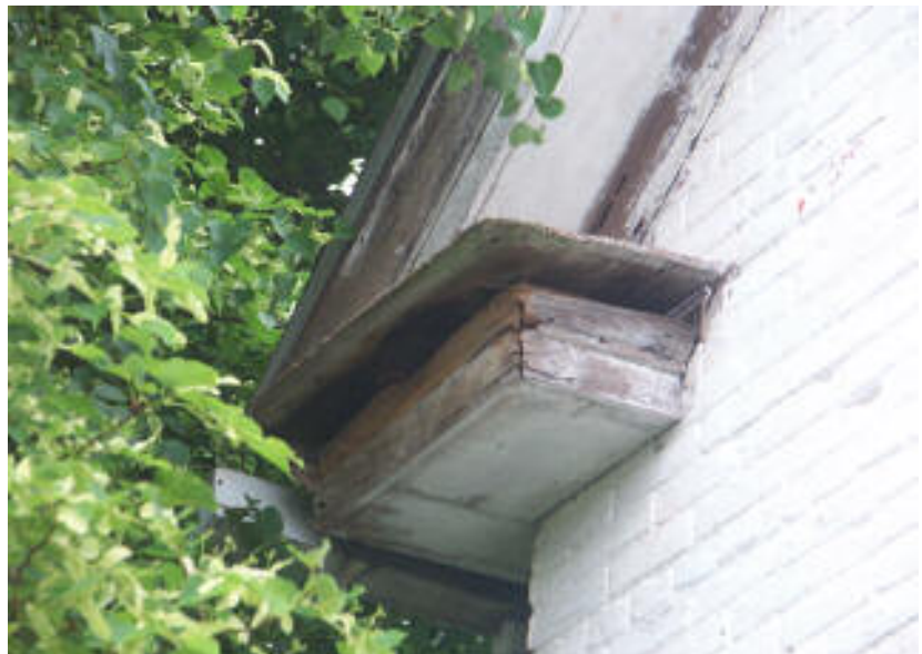
Photo 6. Detail of deteriorating cornice on south end of center section.
