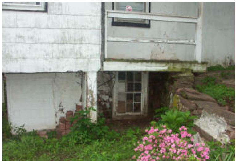
Photo 10. Detail of porch on north end of north section over original basement window.
